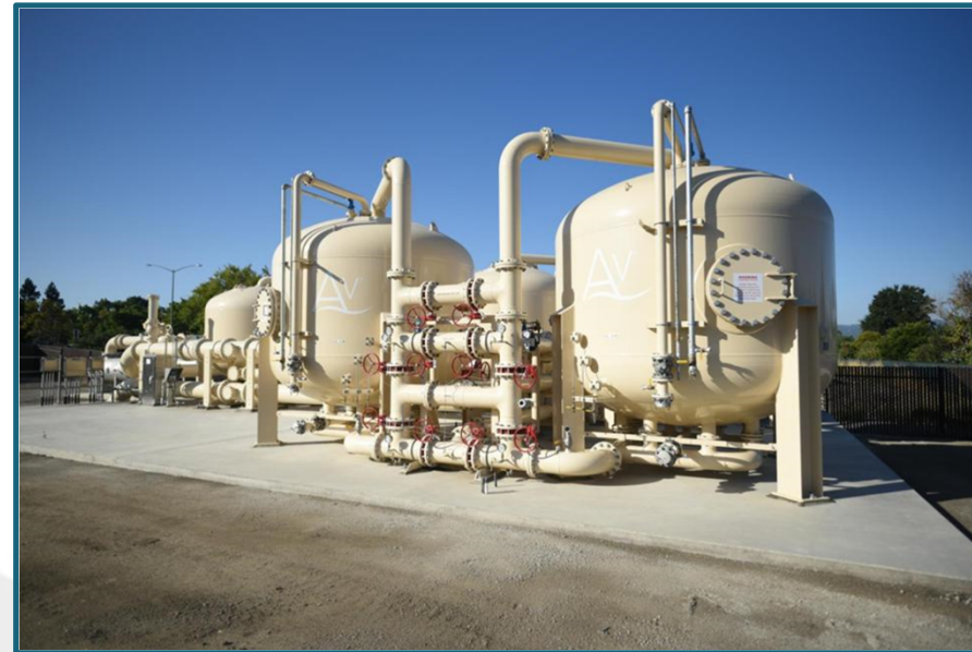
Photo: PFAS Ion Exchange Plant for City of Anaheim
