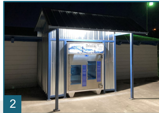
Photos: 1) Point of Use Installation and 2) Drinking water vending machine installed at Pixley Public Utility District
